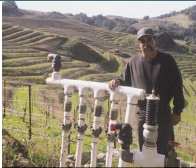
Samuel Félix in 2000 next to the valves, above, and, a drip line, left, of the system irrigating the Napa, California, vineyard where he works. Applying this technology to his orchard in Los Haro, Félix installed the most sophisticated drip irrigation system in Mexico.
